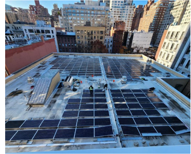
The installation of solar panels at J.H.S. 167 Robert F. Wagner in Manhattan.
